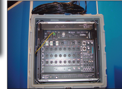
Figure 2.99 Fiber I/O in a flight pack. This system is configured to support an HD or SD camera in a very remote location, along with a number of microphones, intercom and a couple of video feeds back from the truck. The yellow cable is the fiber back to the truck.
