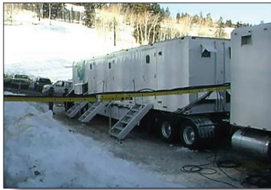
Figure 2.95 A compound at the Olympic Winter Games, using a ladder as a makeshift cable tray. Fire marshals had decreed that no cables could be run on the ground. (Source: John T - NEP)
